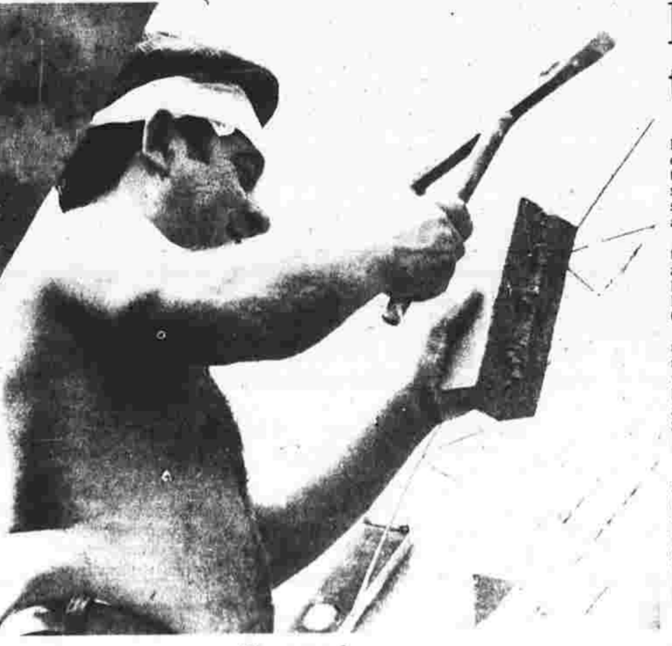
Hot work — Arello Birano, a mason, lays brick on an addition to Multi Circuits Inc., Harrison Street, Manchester, during Monday's hot and humid summer weather. (Herald photo by Pinto)
